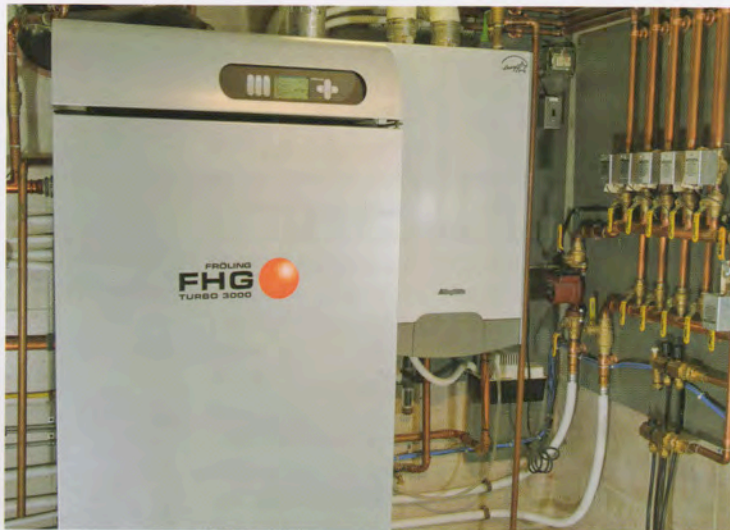
The wood gasification boiler stores excess heat in tanks, greatly increasing the wood heat utilization in the shoulder seasons.
