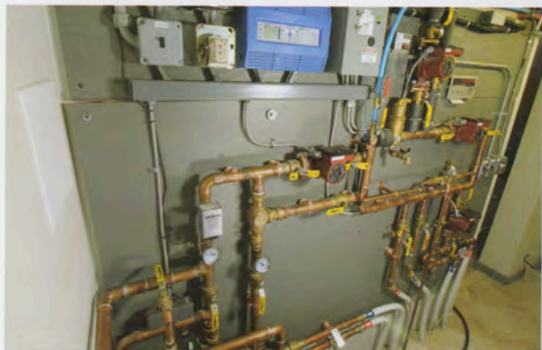
The homeowner describes the mechanical room as “absolutely beautiful.”
